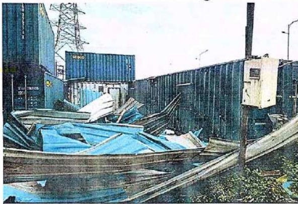
M/s Regal Shipping & Marine Services Pvt.Ltd. (Ziya Container Yard)- 3 Warehouses, Mauje Dhutum, Survey No.4,5,6&7, Taluka Uran, District Raigad. 18.09.2025
