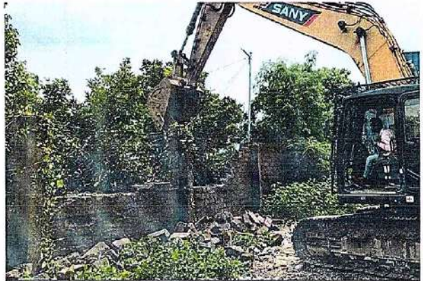
M/s Regal Shipping & Marine Services Pvt.Ltd. (Ziya Container Yard)+ 3 Warehouses, Mauje Dhutum, Survey No.4.5,667, Taluka Uran, District Raigad. 18.09.2025
